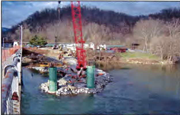
Foundation and Pier Construction from a Causeway Route 61 over the New River
